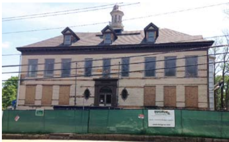
Conversion of the former Blanchard School in Uxbridge into apartments proceeds toward a December completion date.
